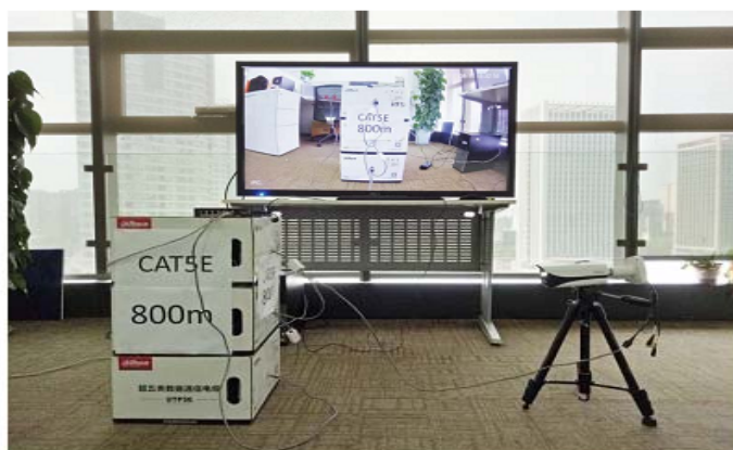
Test of 800m transmission over Cat5E cable
